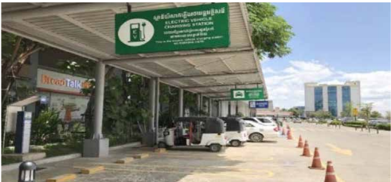
EV Charging Station at a parking lot in a mall in Phnom Penh
